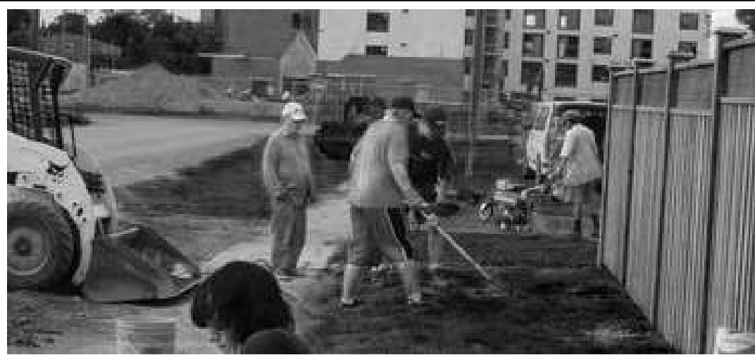
Provincewide, some 50 volunteers from Men's Division International came over a four-week period to lend a hand -- building fence and laying sod.
